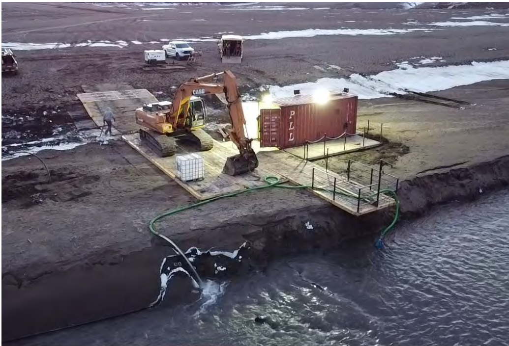
Figure 2: Site overview prior to settling tank installation. Bypass pumping ongoing. Intake overhangs Crowsnest River
