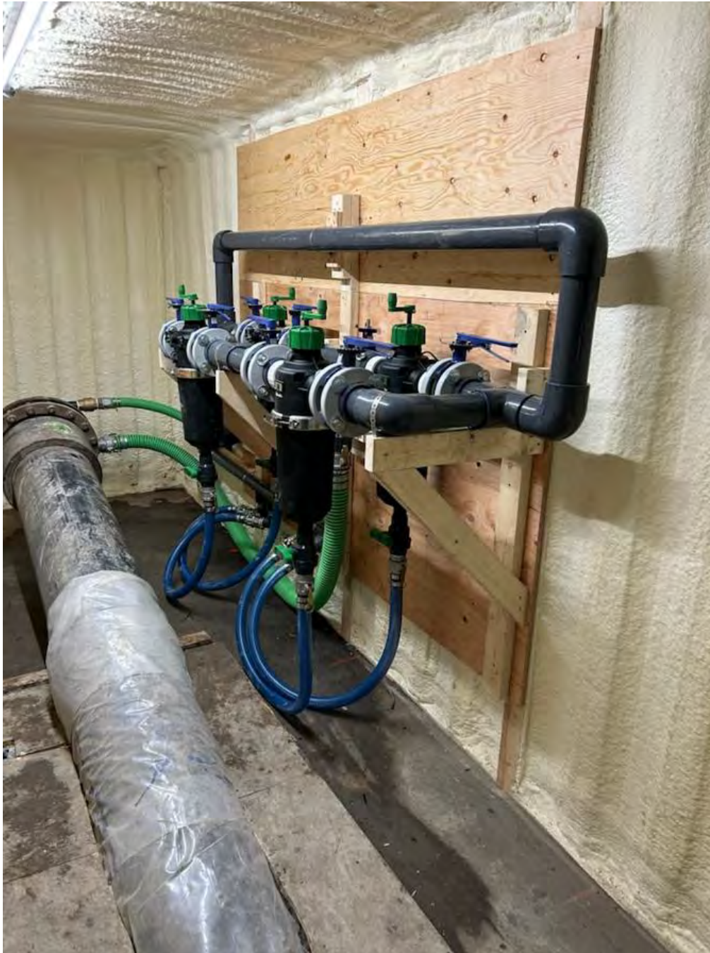
Figure 1: Inside Seacan. Manual pre-filtration setup flowing to existing intake casing
